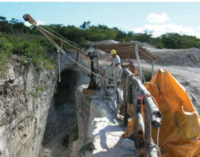
Figure 3. Excavation of the west shaft at the Glorious mine began in March 2006. As of March 2007, the trench and associated tunnels in this area reached a depth of 30 m. Photo by M. Furuya.
