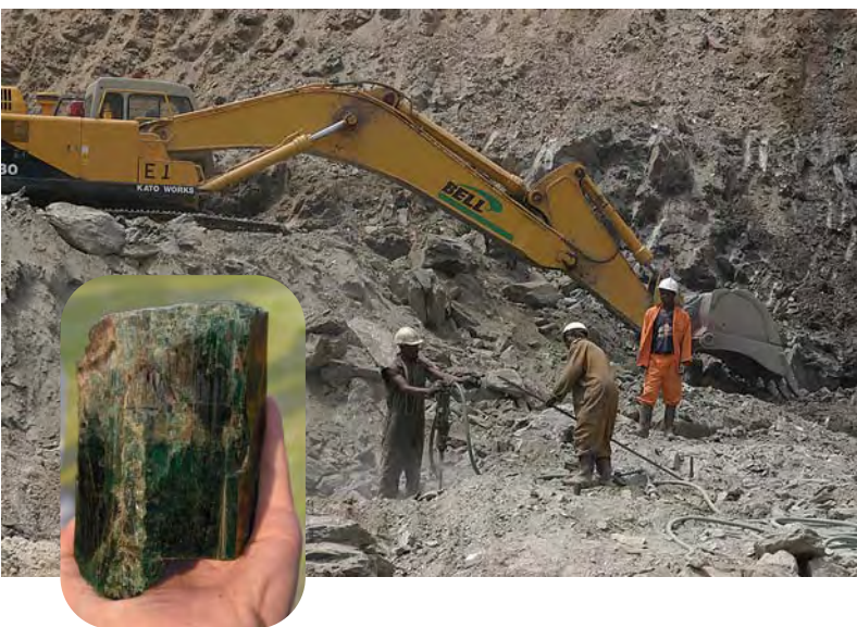
Figure 25. The Chantete emerald mine in Zambia has been worked by mechanized equipment since 2002 in an open pit up to 35 m deep. Occasionally, large emerald crystals are produced (see inset). Photos by Brendan Laurs.
